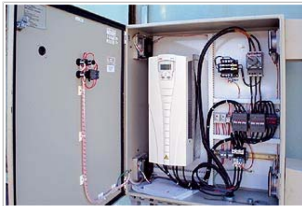
VFD installed at the North Hawaii Hospital. Photo courtesy of Aaron Won
